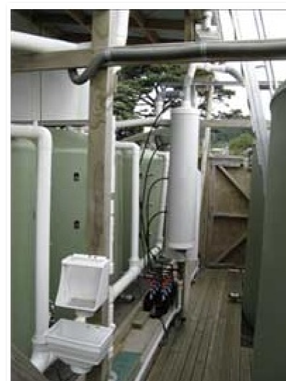
Figure 11: 120L first flush diverter
