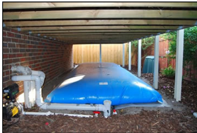
Figure 3: Bladder tank under a deck
