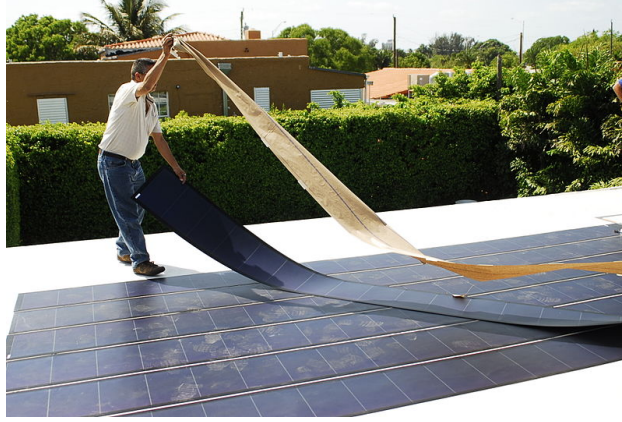
Figure 1.1: Final installation and layout of Uni-Solar Ovonic's Thin Film Flexible Solar PV panels. Photographer: Ken Fields.
