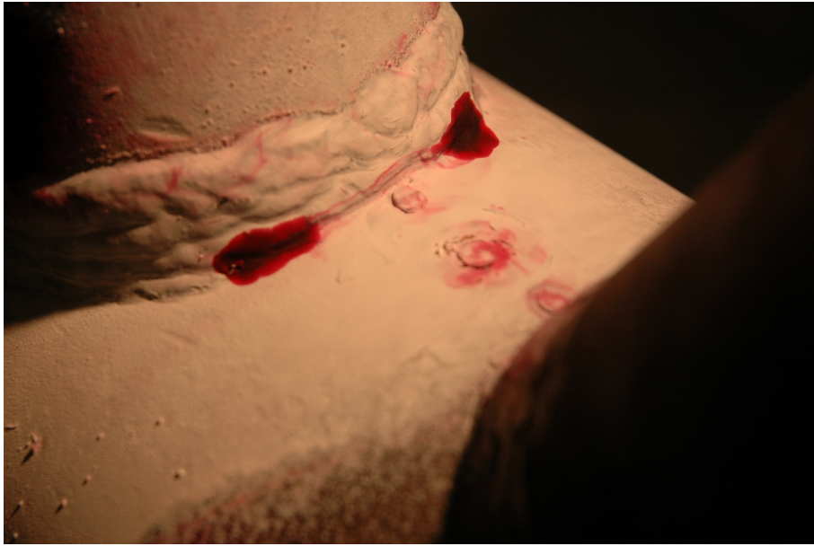
Figure 6.7: A crack revealed (in red) by the dye penetrant technique.
