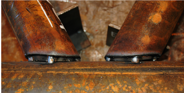
(b) Backing rings fixed onto the chord member by four welding points, and brace extremity positioned over them before welding.
