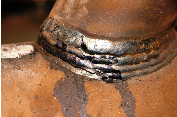
Figure 6.24: The critical crack obtained in joint S7-3S.
