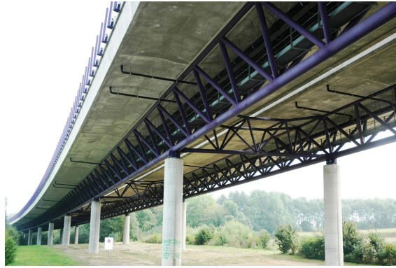
(a) Lully viaduct (canton of Fribourg, Switzerland) composed of two tubular space trusses with KK-joints (typical span 42.75 m, total length 970 m)
