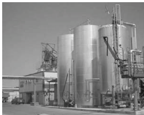
Fig. 4. Insulated tanks used to store bitumen at COLAS premises in Geneva.
