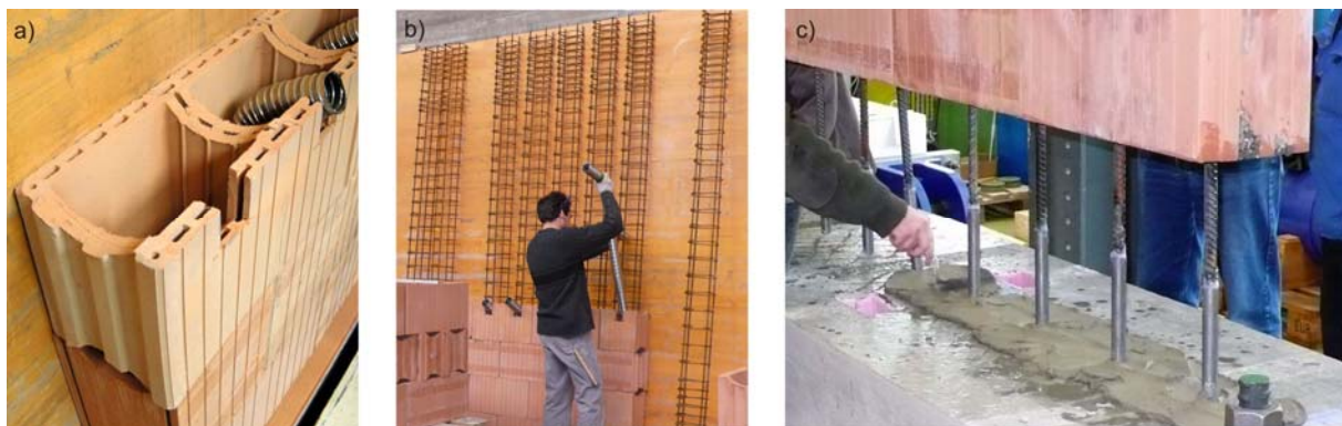
Figure 1. Hollow brick from the UNIPRETON system (a), construction of test units in the precast shop (b) and connection detail when assembling Test Unit BMW1 in the laboratory (c).
