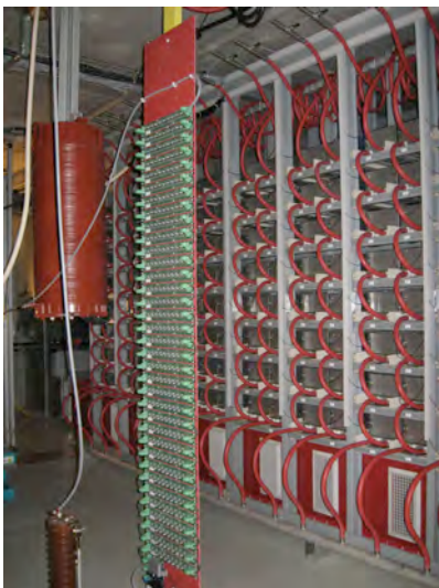
Fig. 4.3.3 Front view of the 128 power modules placed in an isolated frame and cooled down with demineralised water.
