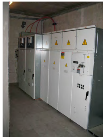
Fig. 4.3.4 AC 20 kV cells, including the start-up system limiting the transformer inrush current to the nominal value.
