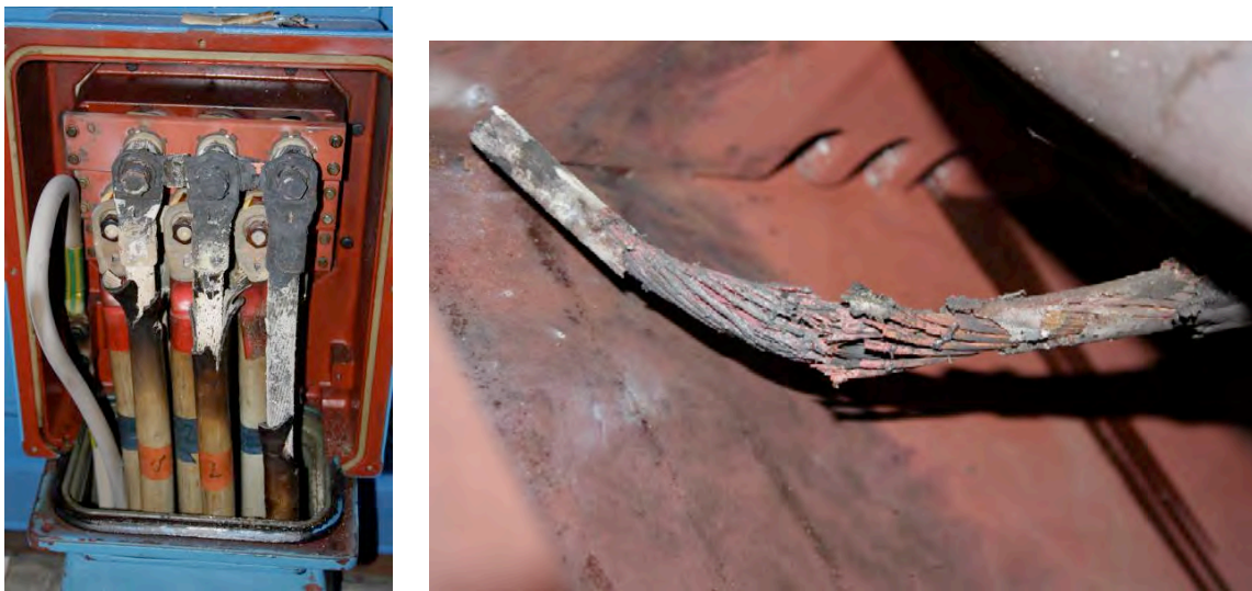
Fig. 3.6.1 Damage of the electrical engine due to over-current in one phase, January 09
