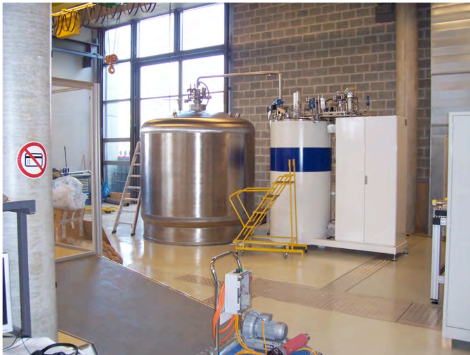
Fig. 3.7.6 Liquid Helium refrigeration system in the test facility hall (0 level). On the right: Helium liquefier (LINDE L140) with a liquefaction capacity of 45l/h without LN 2 pre-cooling and 78 l/h with LN 2 pre-cooling. The liquefier includes a Helium purification system and accepts gaseous Helium with impurities up to 15%. The typical impurity level in the recovered gas is below 5%. The liquefier operation is nearly fully automatic and controlled via a computer interface. On the left: 5000l Liquid Helium storage dewar from where the mobile dewars (3x450l, 3x250l, 20x100l, 15x65l) are filled and will be distributed over the entire EPFL campus.
