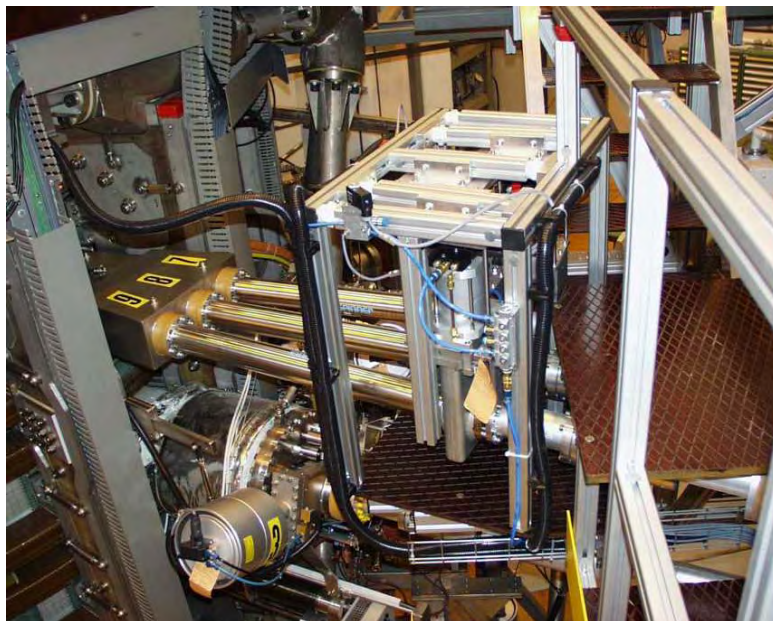
Fig. 3.3.1 Overview of the X3 launcher on top of TCV
