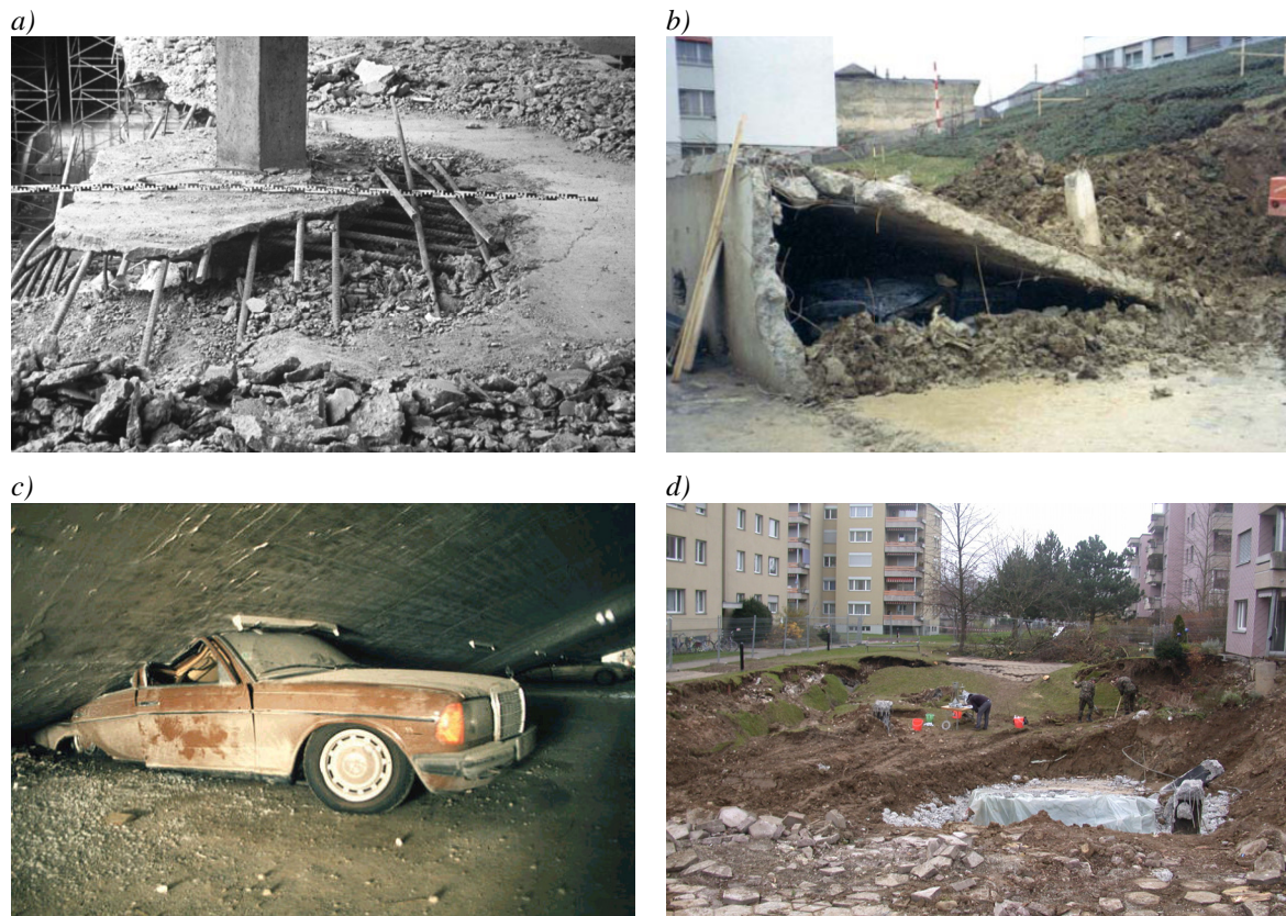
Figure 1.1: Cases of structural collapse due to punching shear failure
