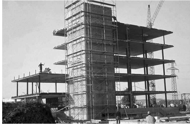
Figure 7.1. Photo of a RC structure with flat slabs and gravity columns and a very eccentric core structure, which is the only member providing lateral strength (photo by the courtesy of H. Bachmann).
