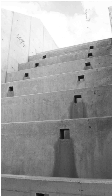
Figure R2 Stepped storm waterway next to railway bridge near Avignon (France) on 20 th September 2000: Pooled steps ( w = 0.4 m, h = 0.7 to 1 m), 45° slope — Note drainage holes (Courtesy Hubert Chanson)
