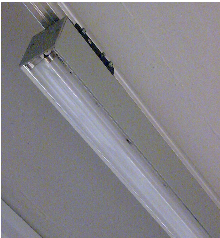
Figure 4.5: The ZEN3 luminaire. - The figure shows a ZEN3 luminaire by Tulux (104) mounted on the test office room's rail system.
