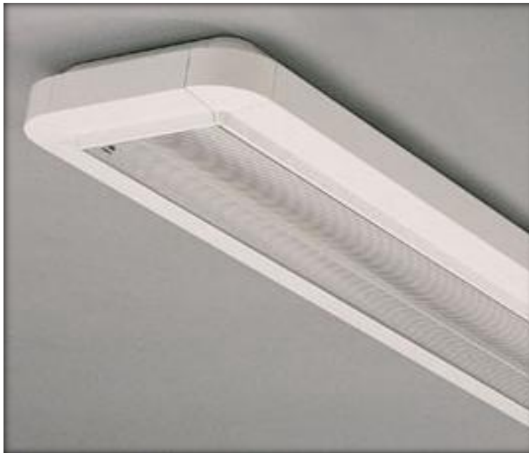
Figure 3.15: The "Lip" luminaire. - The figure shows a "Lip" luminaire by Regent (84) as mounted in many office rooms of the LESO building.
