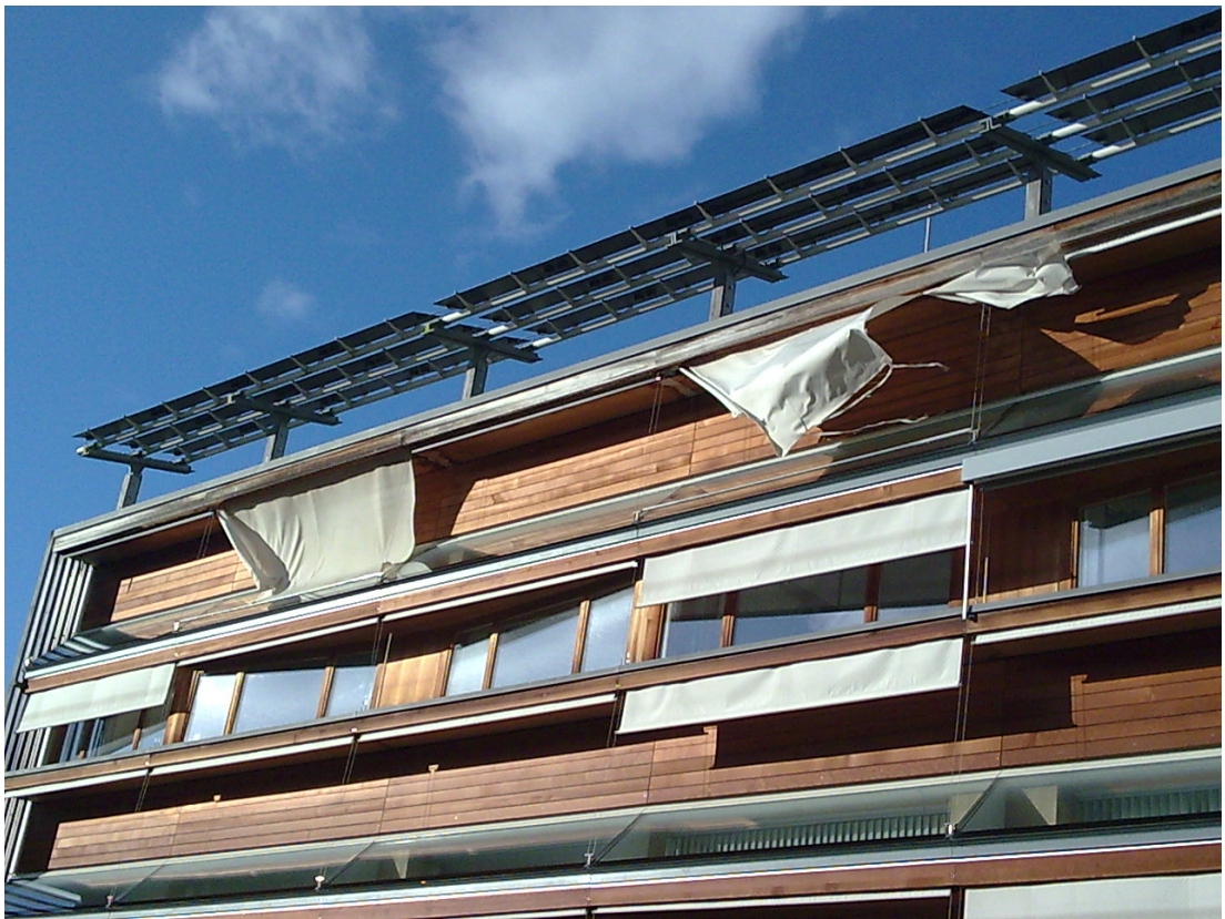
Figure 2.20: Wind damage. - The figure shows wind damage to the window blinds at the LESO building.
