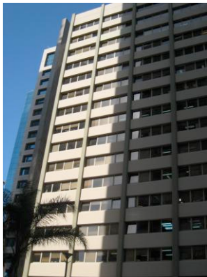
Fig. 1: The South Facing facade of the surveyed building, partly shaded by a high-rise adjacent building.
