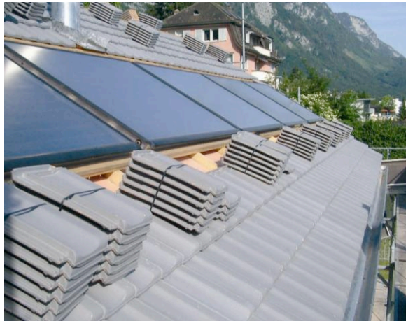
Figure 5: Drain-back solar collectors on the Fehr house. (Photo: H. Fehr)
