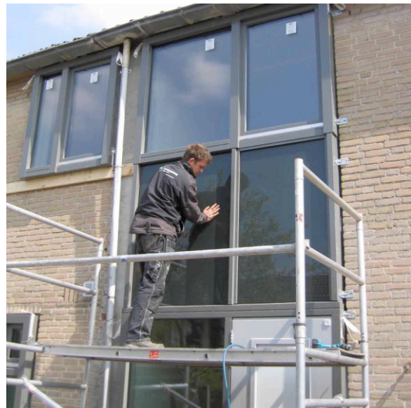
Figure 7: High performance windows being replaced in the Kroeven Project, NL (Erik Franke Architekten)
