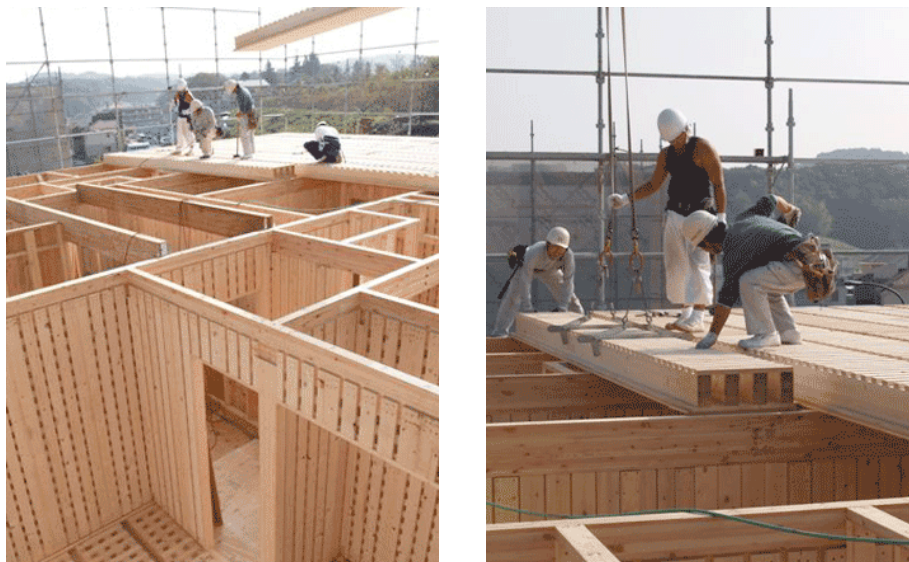
Figure 2: One family house in Aomori (northern Japan), the walls (left) and the roof (right).
