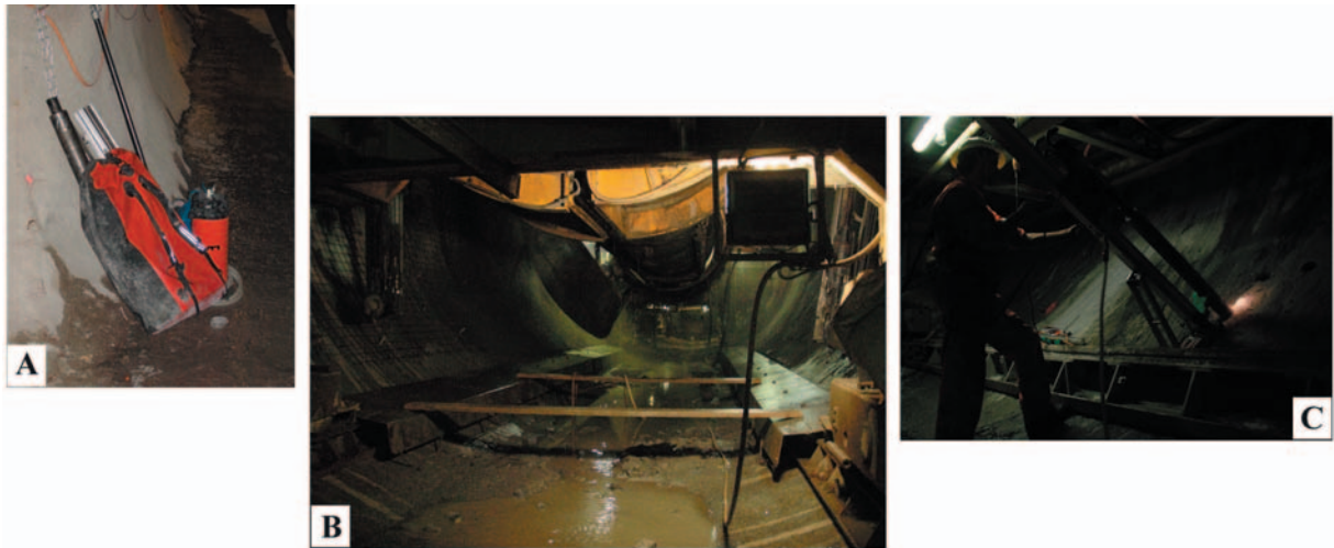
Fig. 5.11 Sampling conditions in the Gotthard base tunnel at Amsteg. Field work has been performed together with Laurent Chaignat and Christophe Veuve in January 2006. A) Material transport. B) Just behind the TBM head. C) Drilling on freshly excavated walls.
