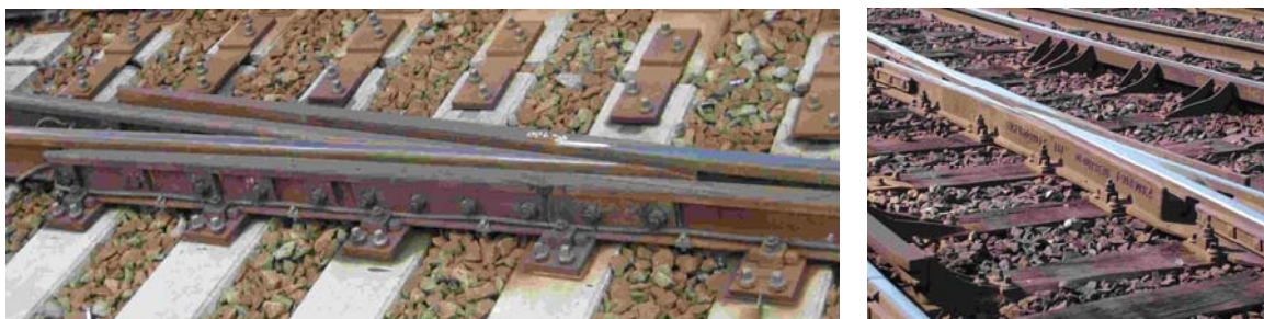
Figure 24 Left: constructed frog type 1 in Rotterdam (NL); right: cast manganese frog in France
