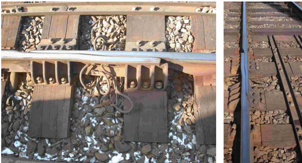
Figure 5 An expansion switch, Lyon (F)
