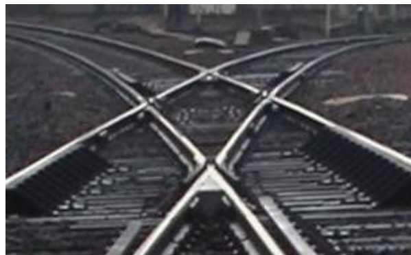
Figure 12 Diamond crossing in the junction of St Benoit (F)
