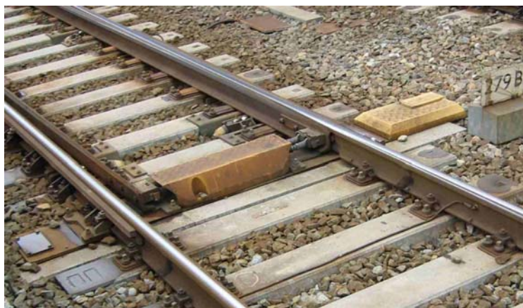
Figure 9 Switch actuator for moving the switch blades, Rotterdam (NL)
