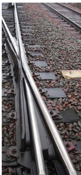
Figure 28 Cast manganese common crossing, Junction of St. Benoit (F)
