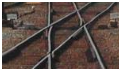
Figure 30 Moveable switch blades in the common crossing part of a diamond crossing, Kijfhoek (NL) 21
