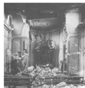
Figure 4.29 : Chancel arch after the main seismic shock in May 1976 [Do 94].
