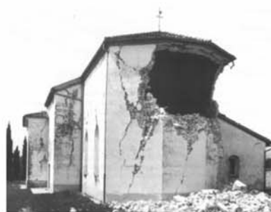
Figure 16.25 : Damage observed on the apse after the earthquake.
