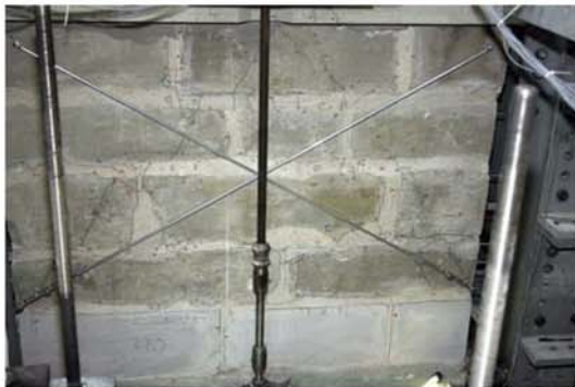
Figure 7.7 : Crack patterns on the west side of the sample for a drift of 8.8‰.
