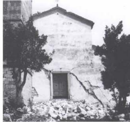
Figure 16.14 : Front wall damaged by the main seismic shock occurred in May 1976.
