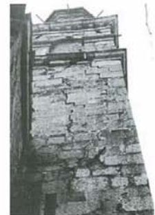
Figure 4.43 : Formation of a crack parallel to the pre-existing fracture caused by a previous earthquake in 1928 (San Marino ad Artegna church) [Do 94].
