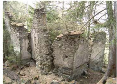
Figure 4.10 : Damaged chapel in Visperterminen; picture taken in 2005.
