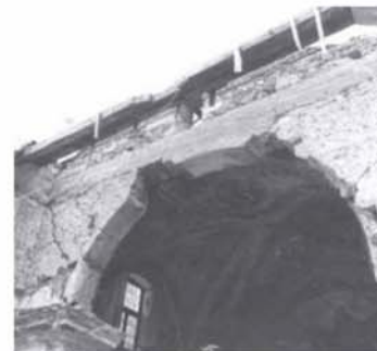
Figure 16.17 : Chancel arch after the main seismic shock in May 1976.
