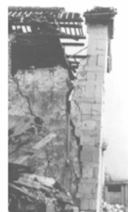
Figure 4.37 : Santa Maria del Fossale: crack between the front wall and the lateral wall mainly due to the difference in masonry and the out-of-plane motion of the front wall [Do 94].
