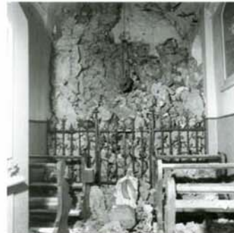
Figure 1.6 : Damage on the Chapel of Lourdes (Sachseln, Obwald) resulting from the earthquake which occurred in the Central part of Switzerland in 1964 [Lau 04]; Photo Reinhard, Sachseln.
