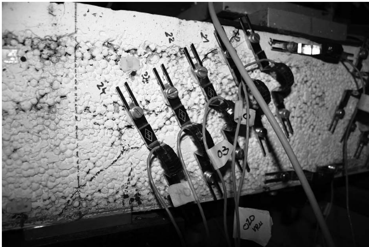
(a) At approximately 165 kN - crack development above O20, O21 and O23
