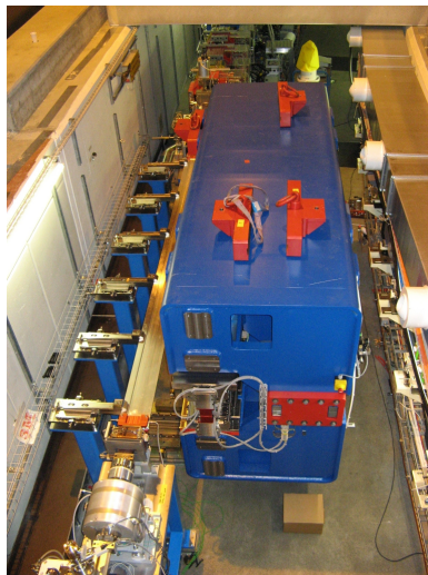
Figure 2.6: Top view of UE44 undulator installed at ADDRESS.
