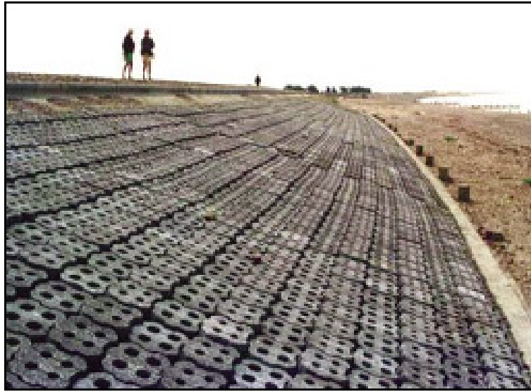
Figure 6.2: Example of a bank protection against flood with a 3D non-woven polypropylene geotextile - [Website of Geofabrics company, England, (2004)]
