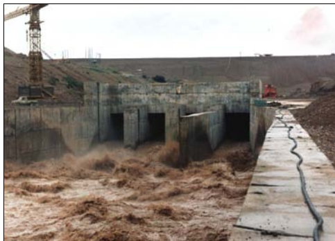
Figure 2: Construction of stilling basin of Karkheh diversion system (above) and a flood about 1800 \text{ m}^3/\text{s} during river diversion (below)
