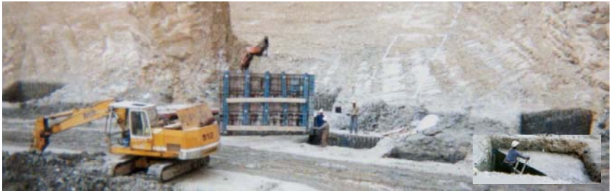
Figure 5: Construction of the concrete prisms downstream of diversion outlets (excavation, formwork and concrete works)
