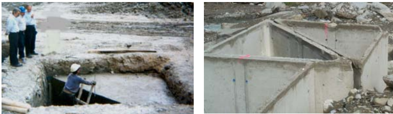
Figure 48: Prisms construction methods, without using sides' formwork and reinforcement (left), precast formwork filled with mass concrete (right)
