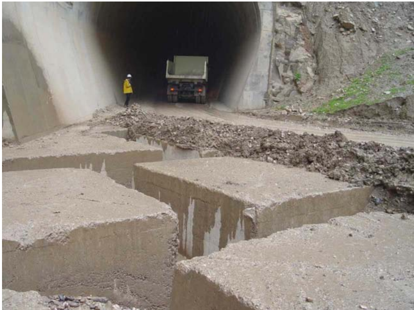
Figure 52: Protection prisms in Seymareh dam project
