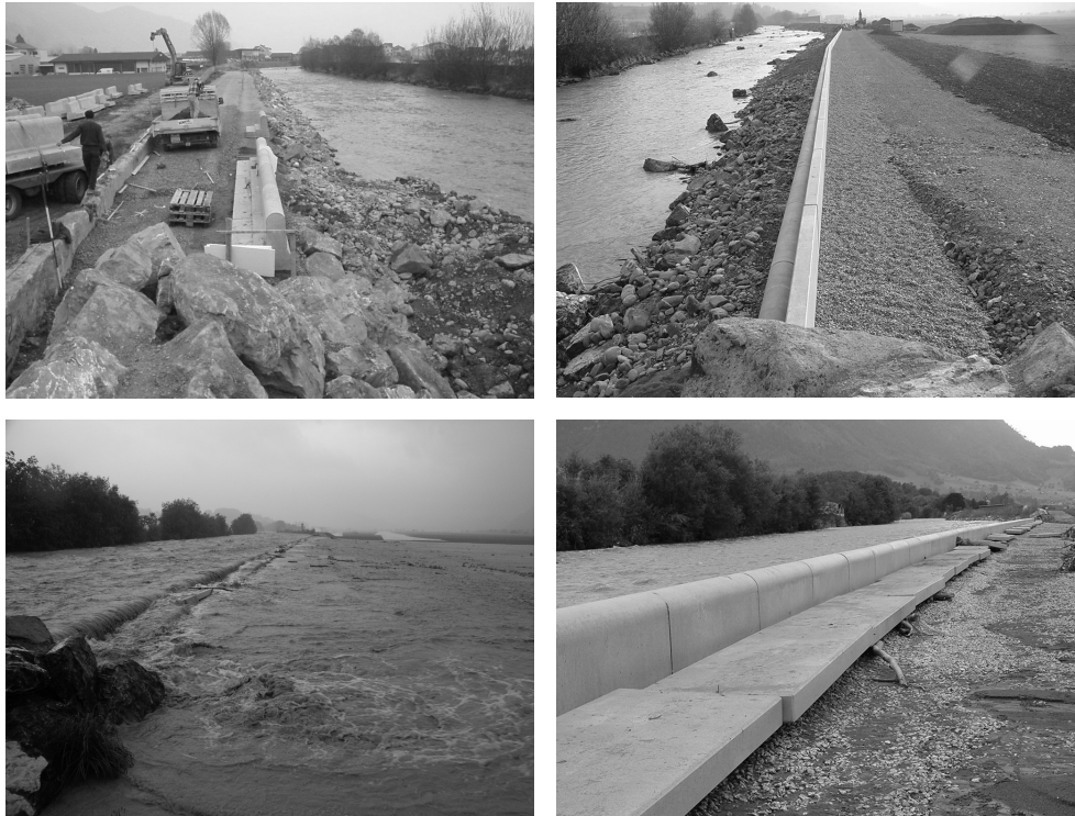
Figure 7.2: Example of a side weir equipped with overturning fuse gates on the river Engelberger Aa, Switzerland (photos: Swiss Federal Office for the Environment - FOEN). Top left: Construction of the side weir. Top right: Side weir equipped with overturning fuse gates. Bottom left: Side weir in operation. Bottom right: Side weir after flood event.
