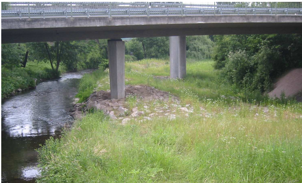
Figure 2.5: Side overflow device on the river Alb, Karlsruhe, south of Germany (photo: B. Rosier).
