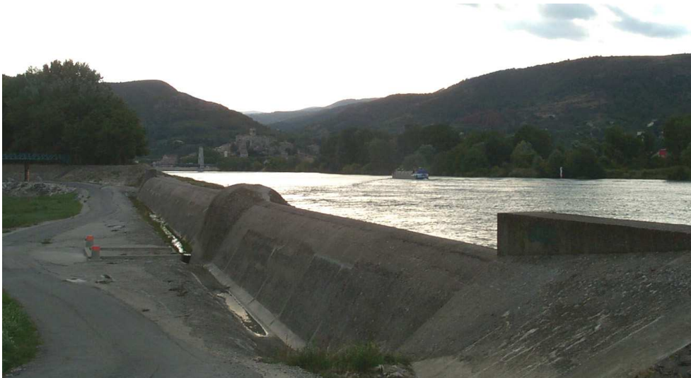
Figure 2.2: Side weir on the lower Rhone river between Valence and Montélimar, France (photo: B. Rosier).
