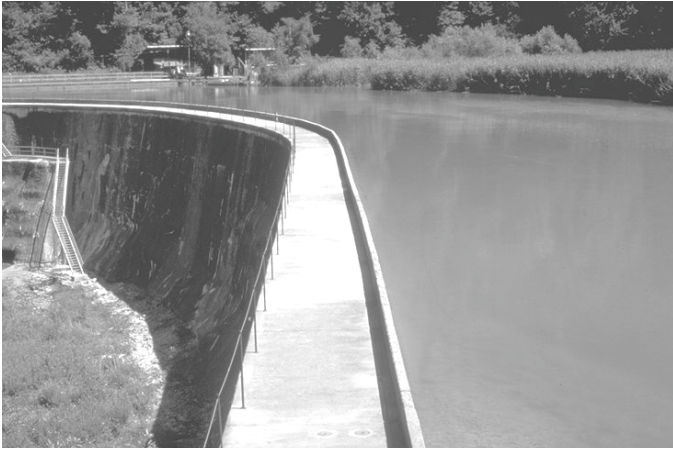
Figure 3. Maigrange dam, 1872, before rehabilitation
