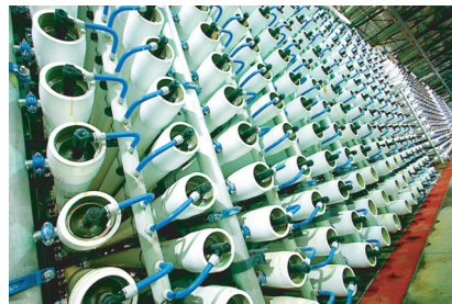
Reverse Osmosis Pressure Vessels
