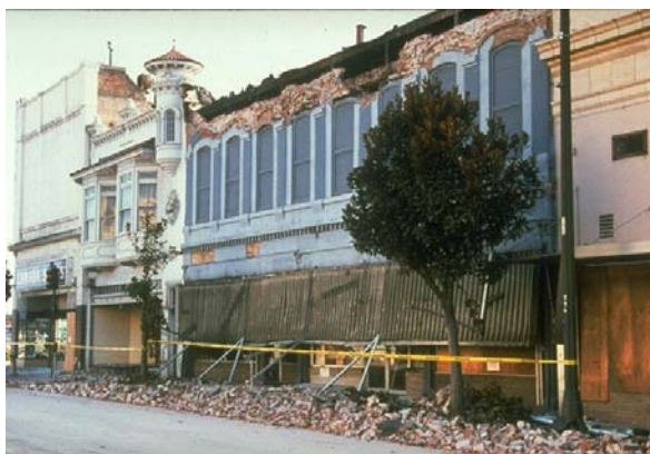
Watsonville, Loma Prieta Earthquake, 1989
