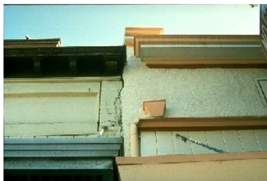
Hollister Area, Loma Prieta Earthquake, 1989
