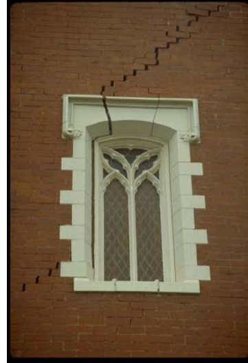
Watsonville, Loma Prieta Earthquake, 1989
