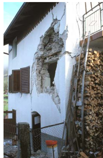
Figure 1.7: Posočje, 1998: disintegration of a stone-masonry wall (Courtesy of Tomazevic, personal communications)
