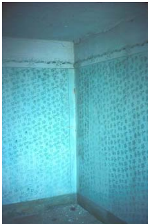
Figure 1.6: Cracks at the joints between walls and wooden floors (Courtesy of Tomazevic, personal communications)
