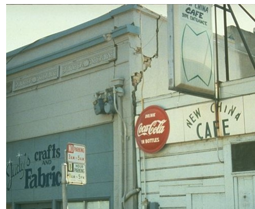
Hollister Area, Loma Prieta Earthquake, 1989
