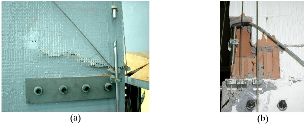
Figure 3.13: L2-GRID-G-F (a) grid rupture in the bottom heel, (b) masonry failure in the bottom toe
